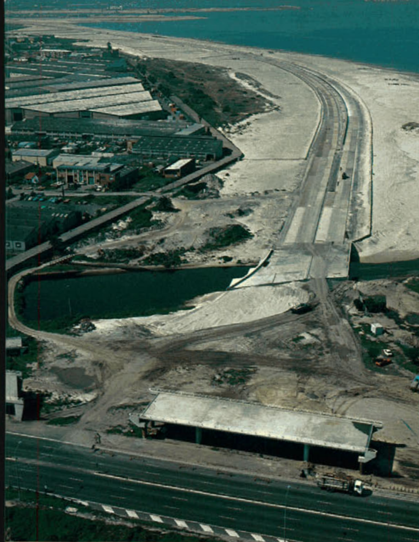
Construction at the north-western end of The Foreshore Road near its junction with General Holmes Drive. The elevated decking in the foreground will eventually carry General Holmes Drive's southbound carriageway over The Foreshore Road.
