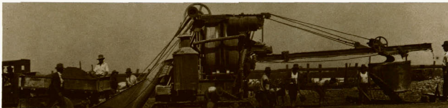
A truck loads the premixed material into the hopper of the paving machine. The travelling bucket at the right pours the concrete onto the roadway.
