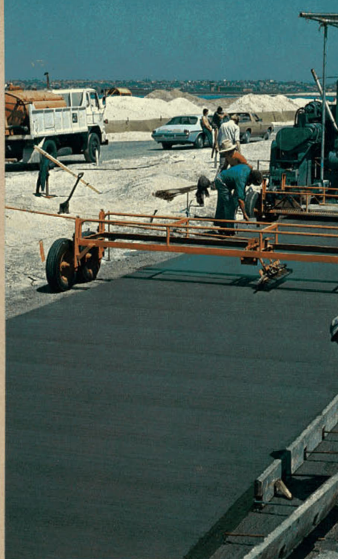
The Stothert and Pitt CPP 60 slip-form paver at work on 140 m 3 /day (8 hours). Pavement texture for maximum skid resistance is achieved by the first trailer to the second trailer. The first trailer held a platform for
