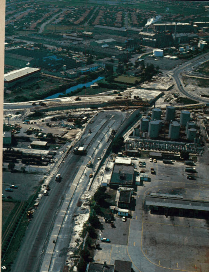
Looking east along the route of The Foreshore Road, showing the railway overpass under construction, the link with Beauchamp Road (on the left centre) and the Caltex depot (on the right centre). The slip-form paver can also be seen.
