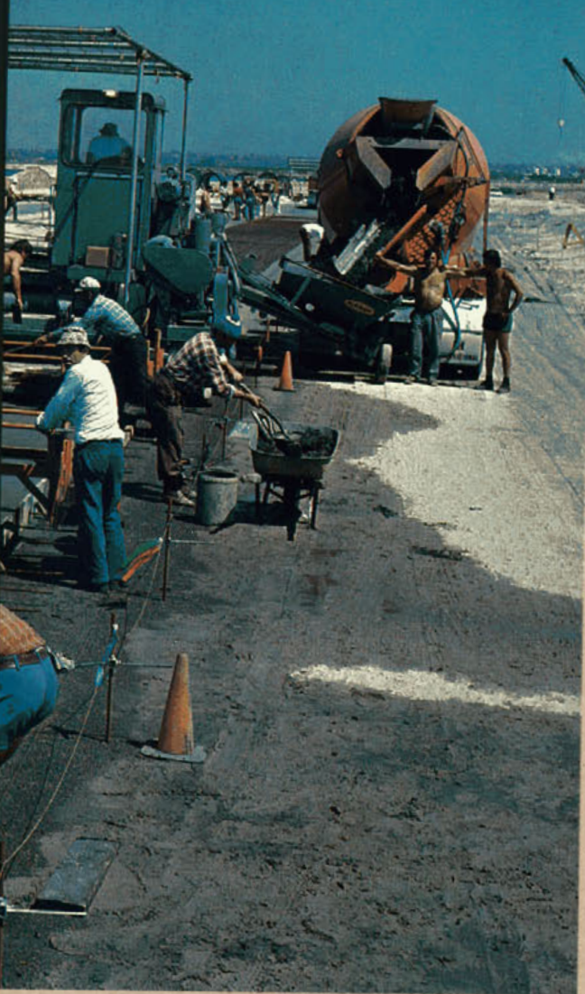
Road. The daily output from this machine averaged 1000 cubic metres. This was achieved by brushing with a wire broom attached to the machine and concrete finishers worked.
