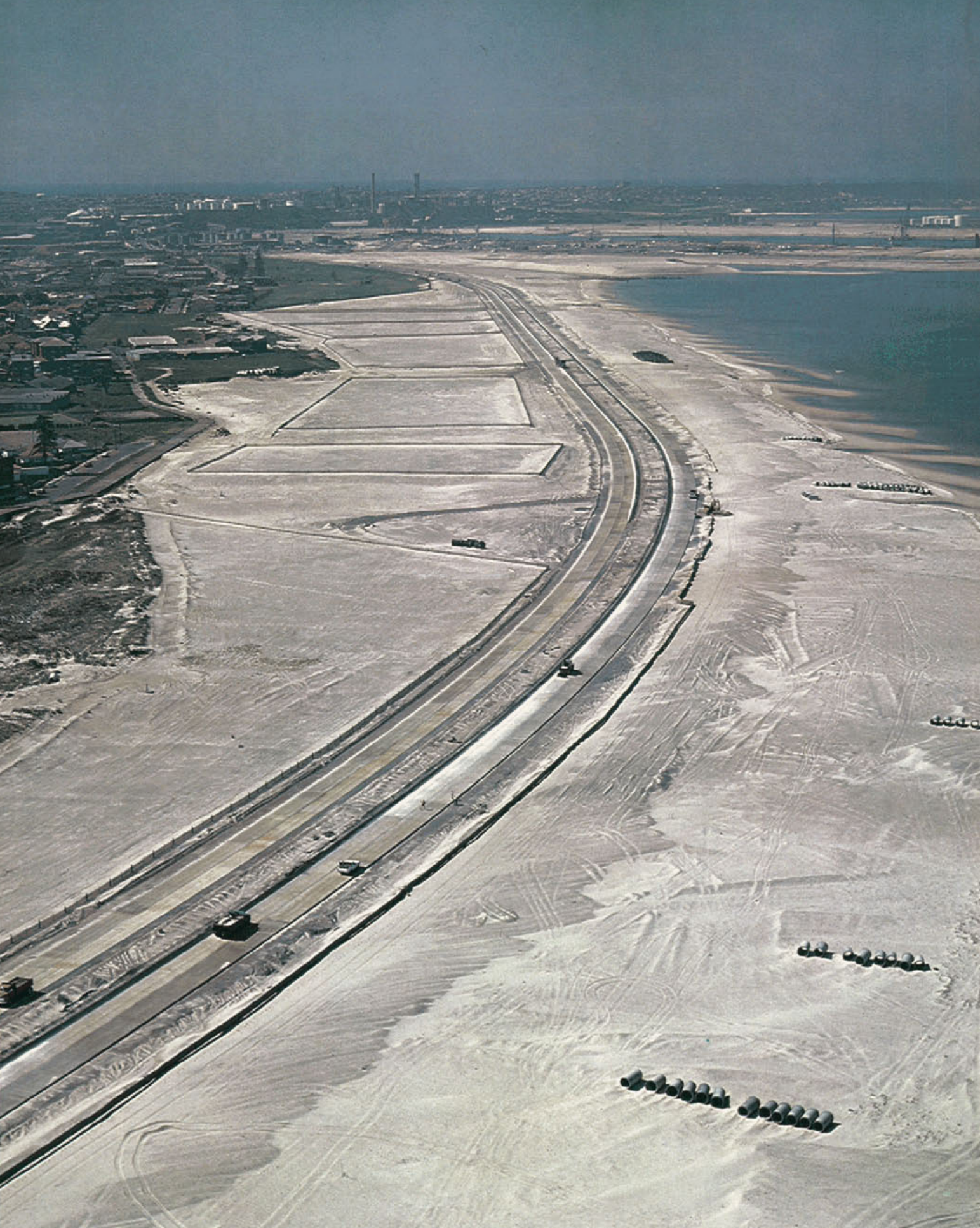
Construction of The Foreshore Road has progressed well. This aerial photograph was taken in March this year.
